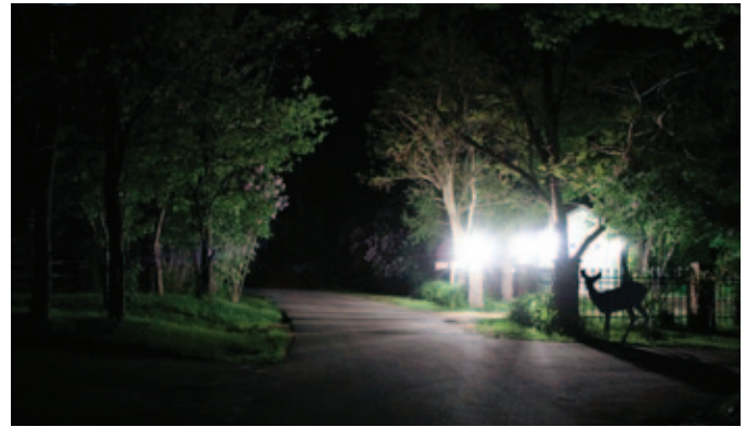
Figure 9 — Aesthetic Lighting at Rural Home. This image was taken at 3 a.m., when the homeowners were absent. The 750 W lamps over-illuminate the entrance and obscure hazards and wildlife along the road. The light attracts vandals and thieves by putting the property’s outdoor furniture and equipment on display. The better it looks to the owners, the better it looks to “ne’er-do-wells,” and they won’t need flashlights to do their nasty deeds.
